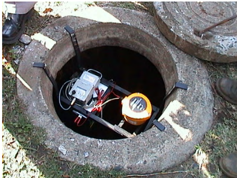
Photo 2: Ultrasonic Flow Measurement and Data Logging at Manhole
