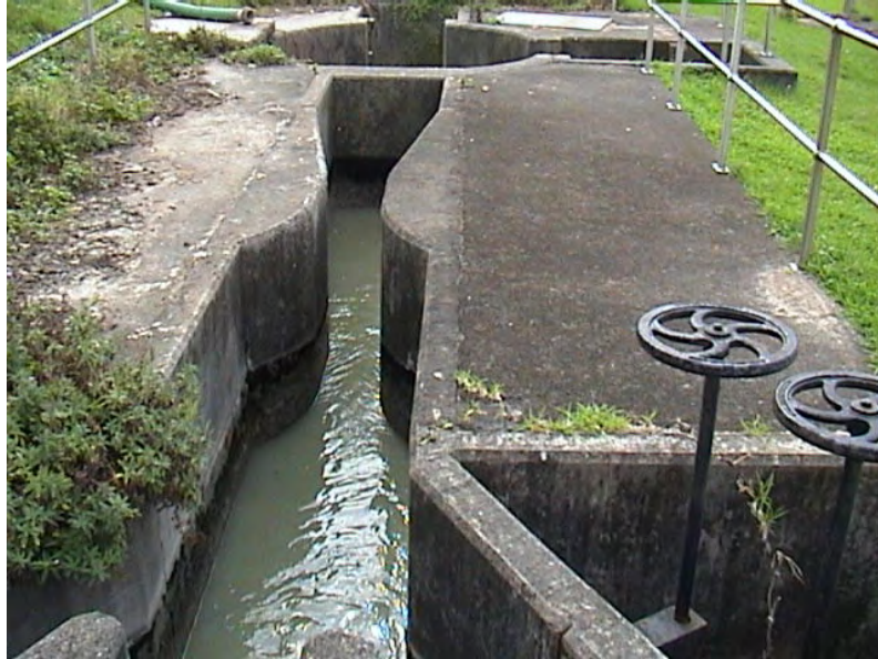
Photo 1: Measurement Flume at STW (outfall)
