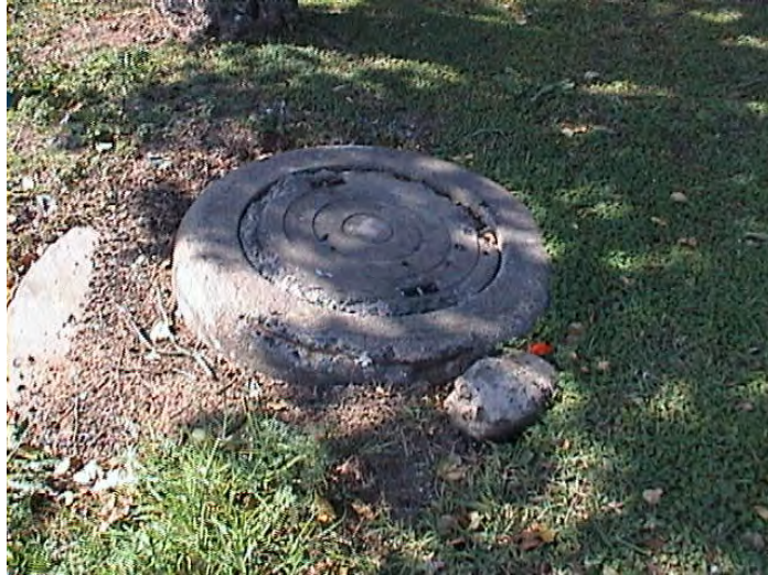
Photo 7: Blow Manhole at PS4
