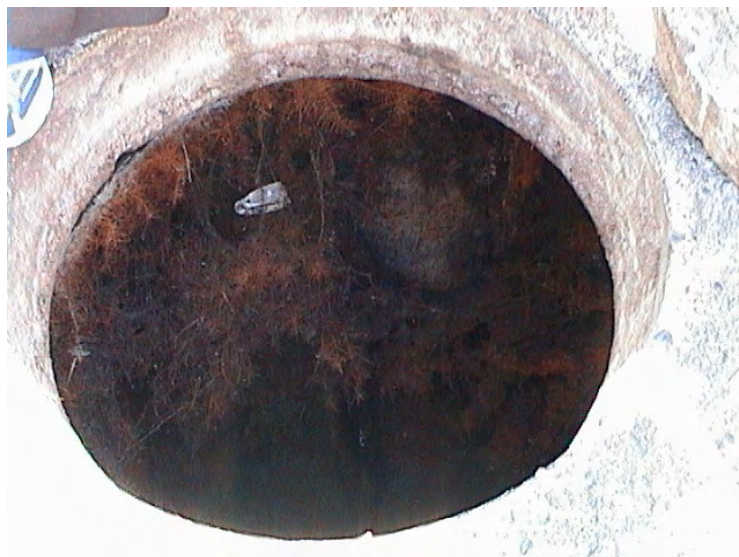
Photo 4: Penetration of roots into Manholes
