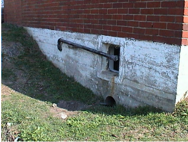
Photo 5: Overflow weir at PS3 into estuary
