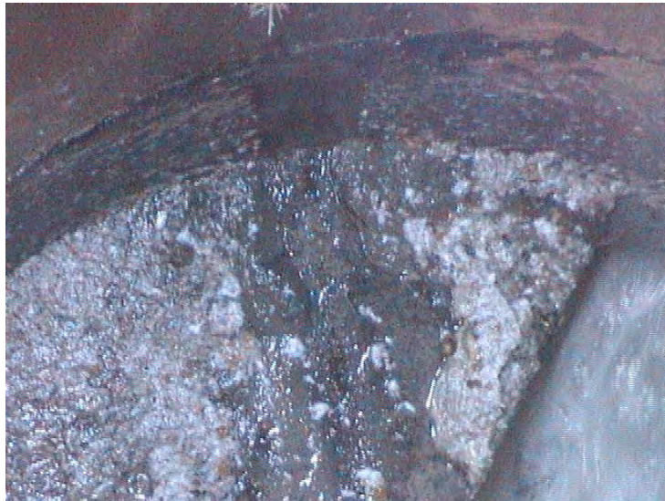
Photo 3: Groundwater Infiltration in Manholes through Benching
