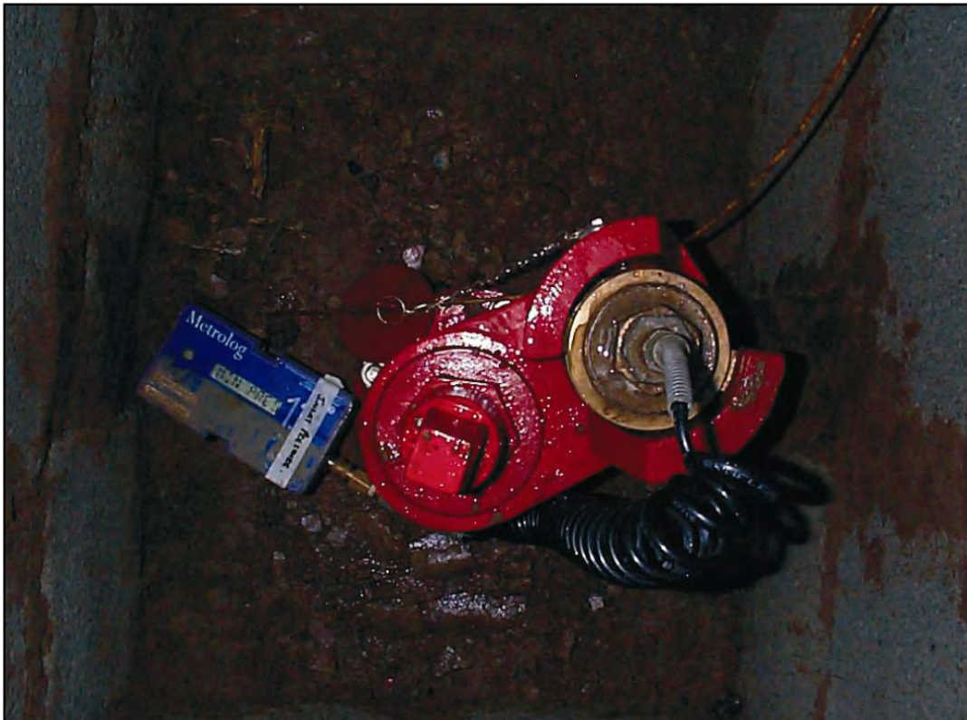
B.6. Logging at a hydrant at the inlet/critical point.
