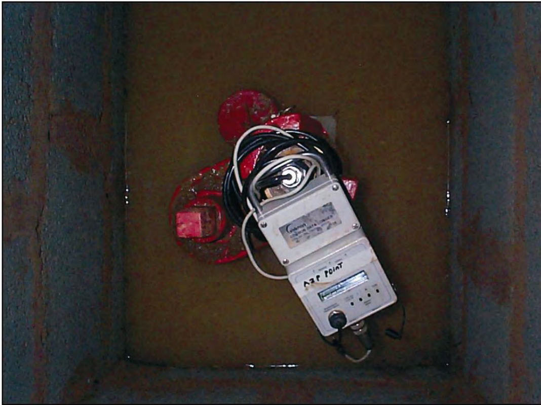
B.7. Logging at a hydrant at the average zone point.
